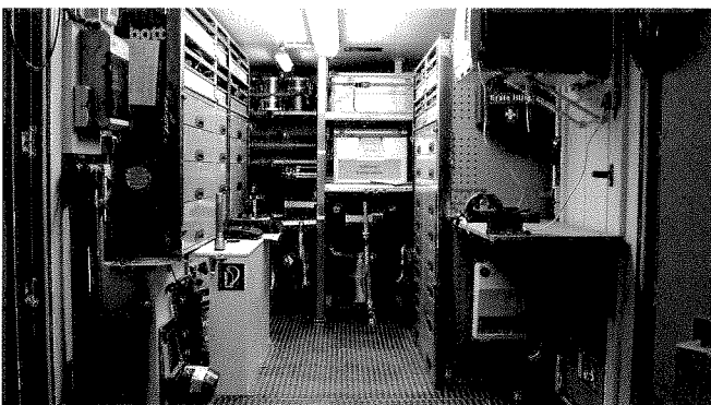
Autonomous workshop with integrated power unit
